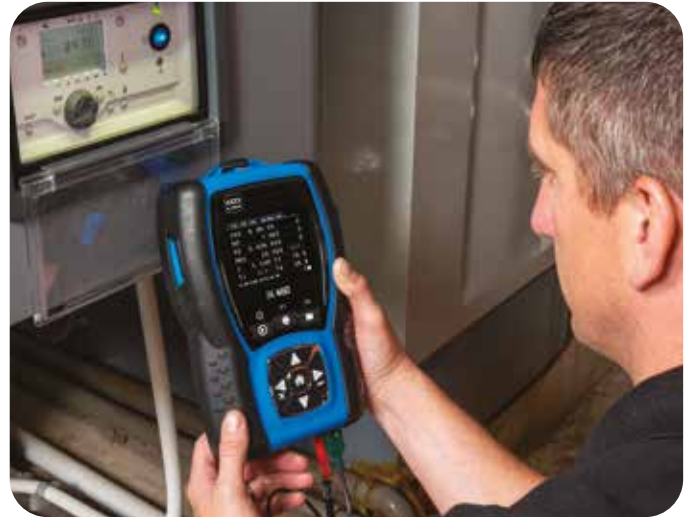
Confirm boiler safety & efficiency
